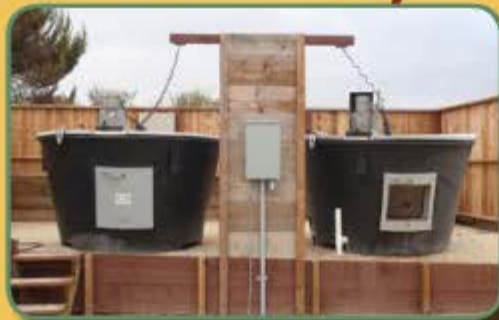
Above: Composters Below: Zero Waste Facility
