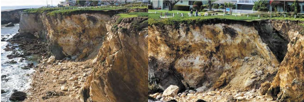
Figure 5-33 Bluff Erosion and Overlying Development at Dinosaur Caves Park in Pismo Beach, January 2010
