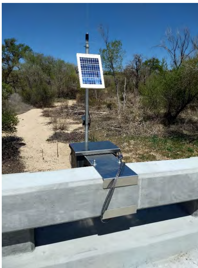
Figure 4. Creston (Huer Huero Creek) radar sensor stream gage installation
