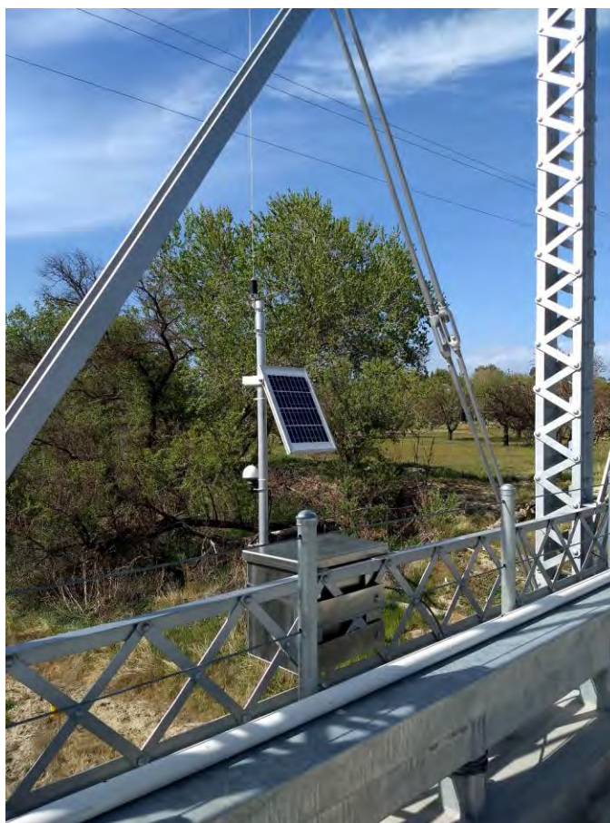
Figure 2. Whitley Gardens (Estrella River) radar sensor stream gage installation
