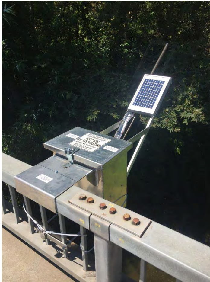
Figure 2. San Luis Obispo County radar sensor stream gage installation
