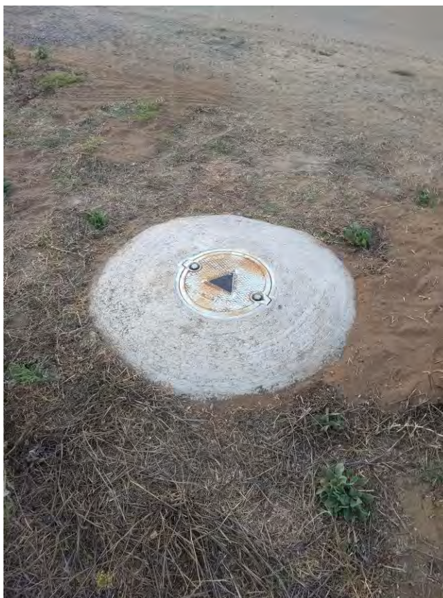
Figure 1. Typical 12-inch monitoring well box
