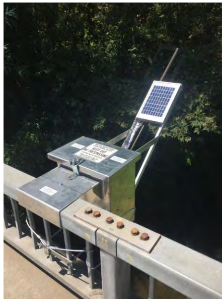
Radar Sensor Stream Gage: County of San Luis Obispo
