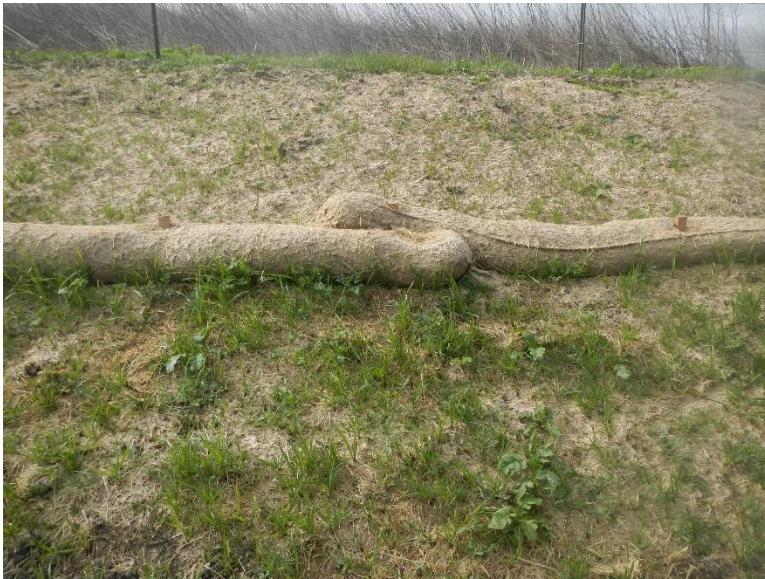
Sediment Control perimeter protection (Straw Wattles)
