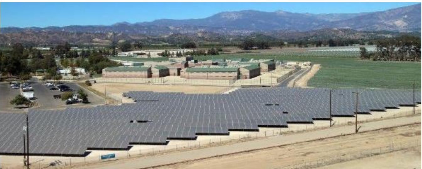
1 MW Ground Mounted solar array at the Todd Road Jail Facility in Santa Paula. Photo courtesy of Ventura County.
