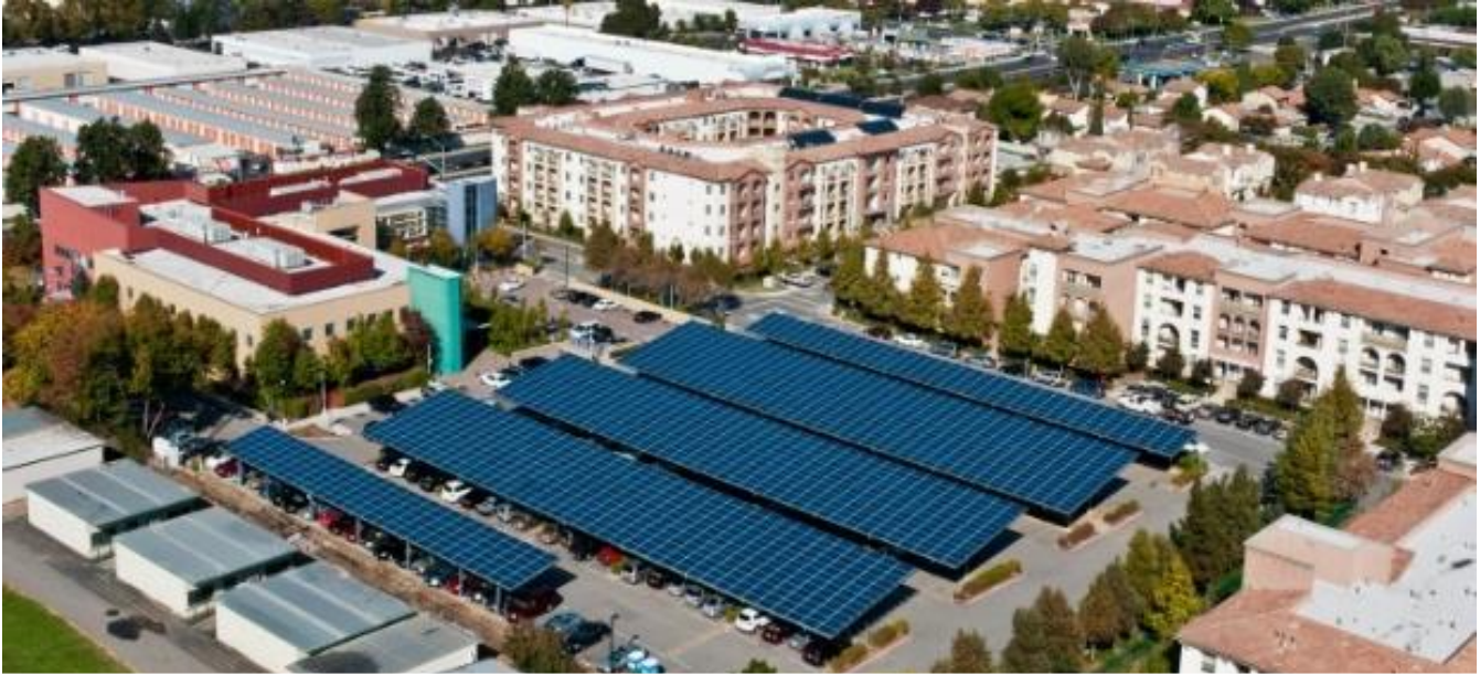
441 kW carport PV installation at the Valley Health Center in San Jose. Photo courtesy of Santa Clara County.
