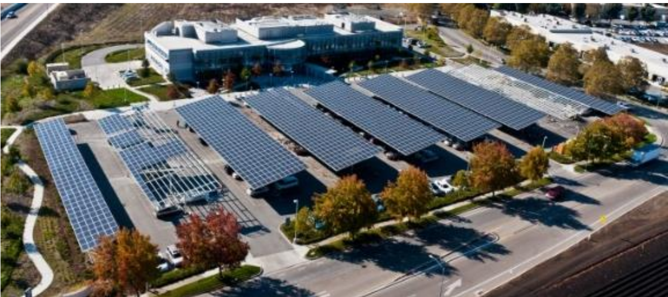
706 kW carport PV installation at the Gilroy Health Center. Photo courtesy of Santa Clara County.
