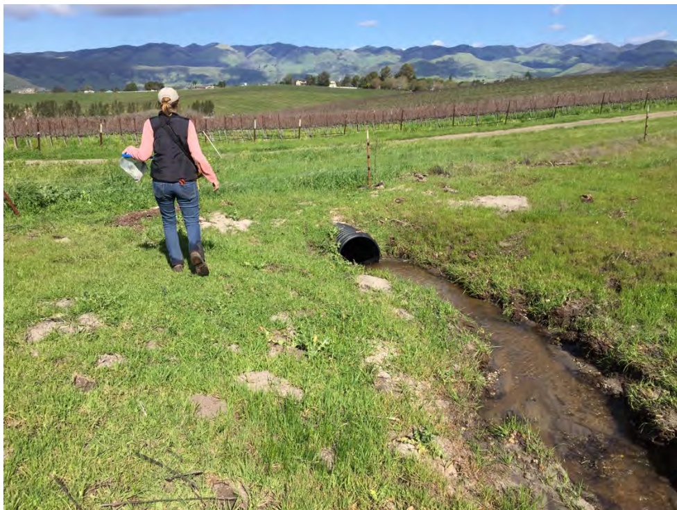
Photo 4: View northwest of the southeastern drainage where it enters a culvert running under the vineyard to the north. This drainage flows into the tributary to Davenport Creek.
