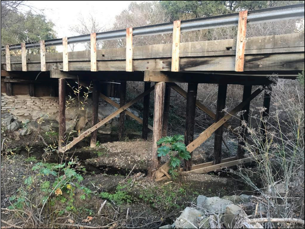
Photo 1: Villa Creek Road Bridge over Villa Creek, facing west. All work will occur on the western abutment and outside the stream channel.
