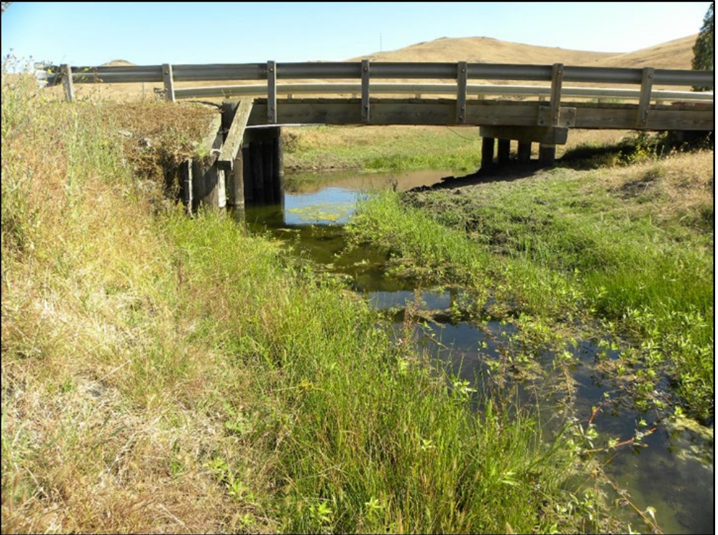
Photo 2: Picachio Road Bridge over an unnamed tributary to Cayucos Creek, facing north. Work will occur on both abutments and the stream will be diverted if water is present.
