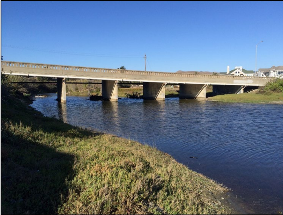
Photo 3: North Ocean Avenue Bridge over Cayucos Creek, facing northeast. Work will occur along the side of the bridge visible here with a complete containment system – no ground disturbance.
