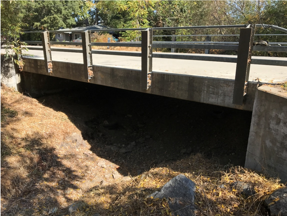
Photo 5: Encina Avenue Bridge over Yerba Buena Creek, facing northeast. Work will occur on the top and bottom of the bridge deck – no ground disturbance.
