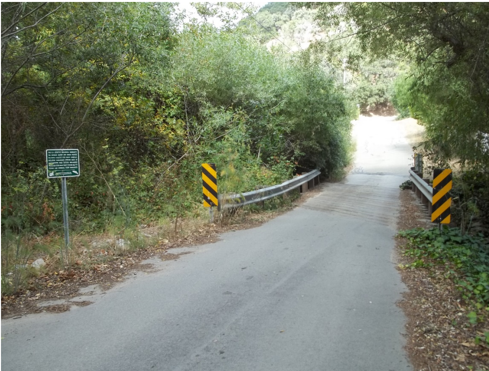
Photo 6: Pippin Lane Bridge over the unnamed tributary of San Luis Obispo Creek, facing north. Work will occur on both abutments and the stream will be diverted if water is present.
