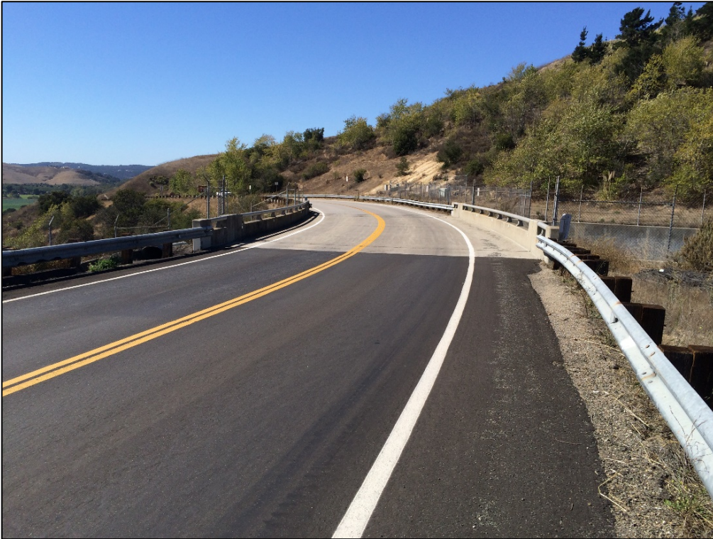
Photo 7: Lopez Drive Spillway Bridge is located on top of the Lopez Dam spillway. Work will occur on the top of the bridge deck only – no ground disturbance.
