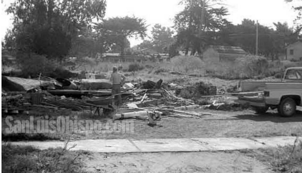
Figure 4.5-3. Demolition of the Richard Otto house in 1983 (courtesy of the SLO Tribune)
