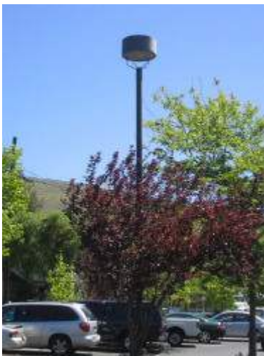
Fig. 7-14 Parking lot light
