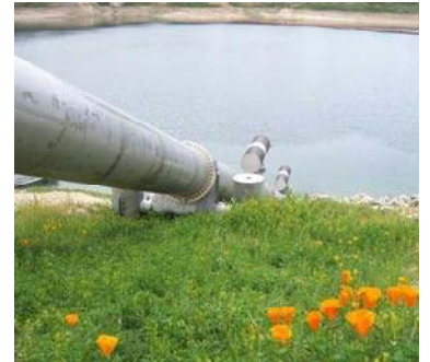
Completed and operational by 2011, the Nacimeinto Water Project increased water supply for many communities in the county.
