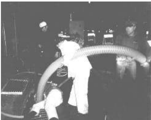
Bleeder line, Farrall Road, Arroyo Grande.
