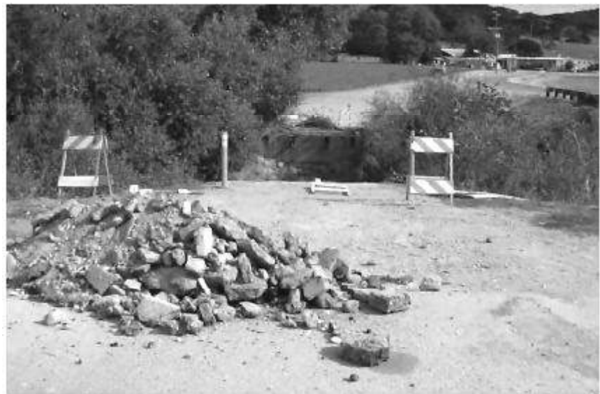
Flooding damaged a bridge over Arroyo Grande Creek.
