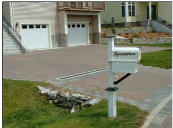
Figure 5.7 Intercepting Driveway Runoff Directing driveway runoff into a vegetated area by intercepting it with a trench drain is one way to reduce the volume of runoff leaving the site during small storms.
