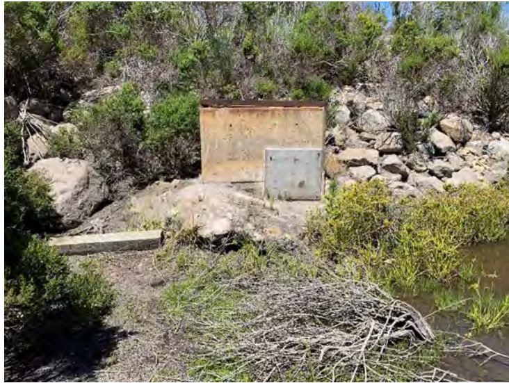
Photo 9: Close-up view of the drainage structure at the south end of the CCC wetlands within the survey area.
