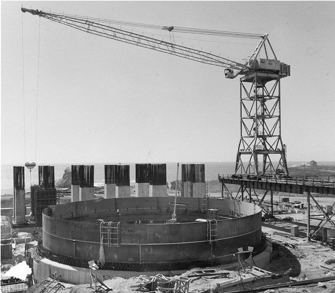
Figure 15. Early progress on the Unit 1 Containment Building and concrete pedestal for the Unit 1 portion of the Turbine Building in April 1970. Source: Pacific Gas and Electric Company.
