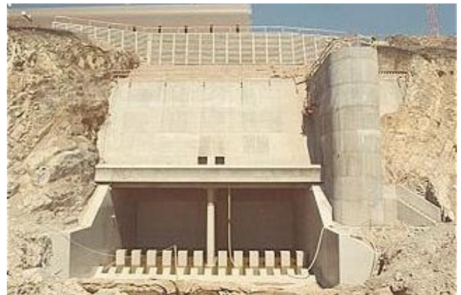
Figure 2: Undated photo of the Discharge Structure's outlet under construction, looking northeast at cove bed with the north half of the Turbine Building visible above. The outlet is currently submerged. Source: PG&E.
