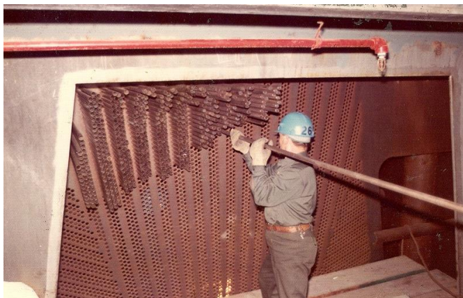
Figure 4: 1972 photo of installation of copper tubing for condenser for Unit 1. Source: PG&E.
