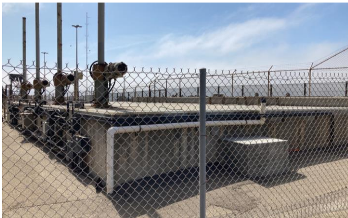
Figure 1: Top of Discharge Structure at ground level looking south. Source: Page and Turnbull, 2021.
