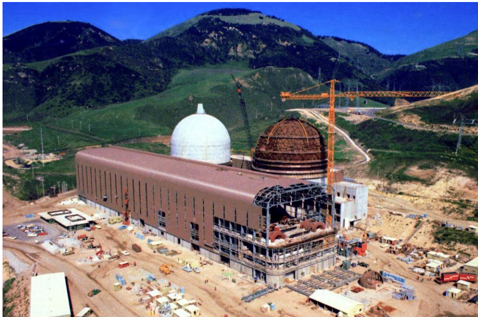
Figure 3: Undated construction photo of south half of Turbine Building nearing completion, looking northeast. Source: PG&E.
