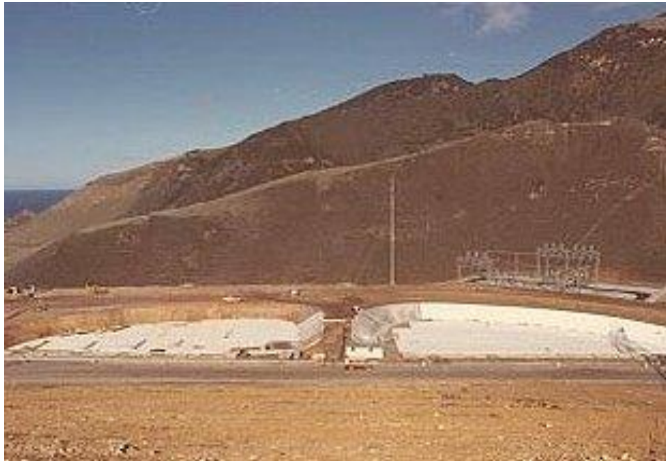
Figure 25. The raw reservoir ponds under construction in November 1972 at the upper terrace above the containment buildings. Source: Pacific Gas and Electric Company.
