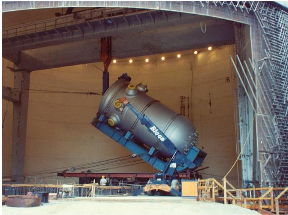
Figure 26. Installation of the Unit 1 reactor vessel within Unit 1 Containment Building in early 1973. Source: Pacific Gas and Electric Company.
