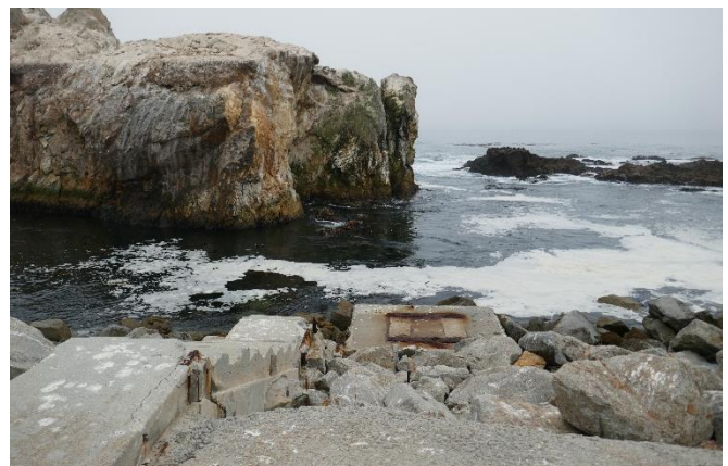
Figure 4: Concrete stairs for ocean side access on south side of East Breakwater, looking southwest.
