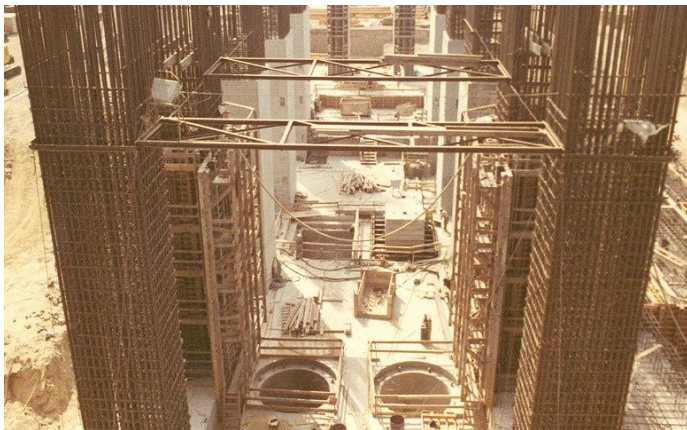
Figure 1: 1972 photo of the ground level of Unit 2 turbine structure under construction, visible are the openings for the intake and discharge tunnels, looking south. Source: PG&E.
