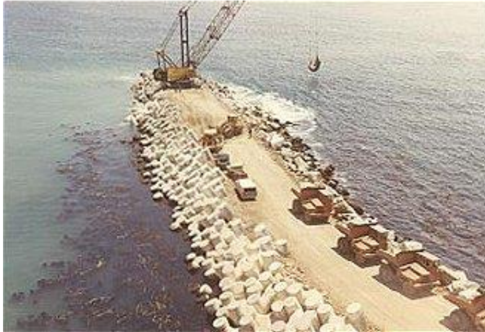
Figure 18. One of the breakwaters under construction in June 1971. Source: Pacific Gas and Electric Company.
