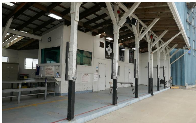
Figure 2: View of exposed interior of Firing Range building, looking north. Source: Page and Turnbull, 2021.
