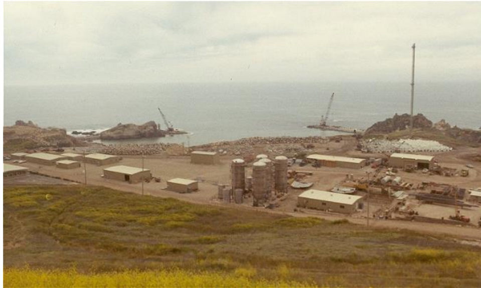
Figure 22. Support buildings and structures in the fabrication yard in April 1971 (currently Parking Lot 6 in Zone 5). In the background, the breakwaters are under construction in the intake cove. Source: Pacific Gas and Electric Company.
