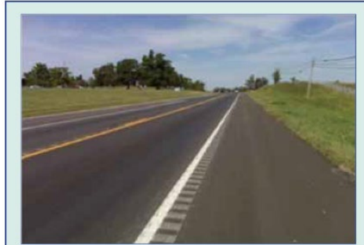
EDGE-LINE RUMBLE STRIP
