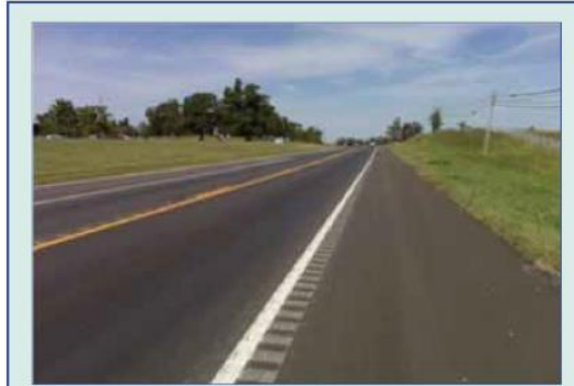
EDGE-LINE RUMBLE STRIP
