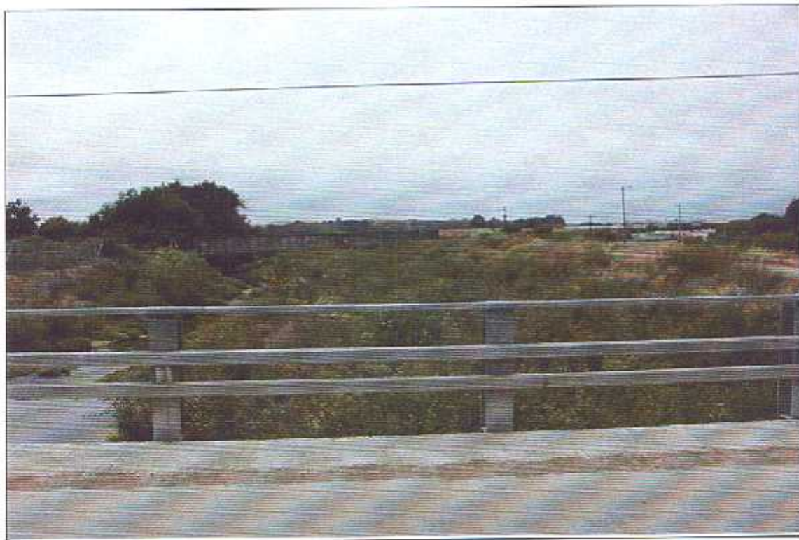
Photo 8 Segment 5. Downstream view of Arroyo Grande Creek flood control channel and railroad crossing from 22 nd Avenue Bridge. Sediment with riparian/ruderal scrub on right in photo is proposed for removal from work area #19.
