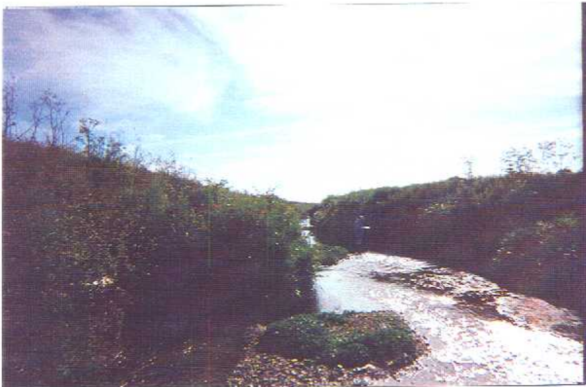
Photo 6: Segment 5. Downstream view of Arroyo Grande Creek flood control channel from access road crossing #3. Sediment with riparian/ruderal scrub along right bank in photo is proposed for removal from work area #15.
