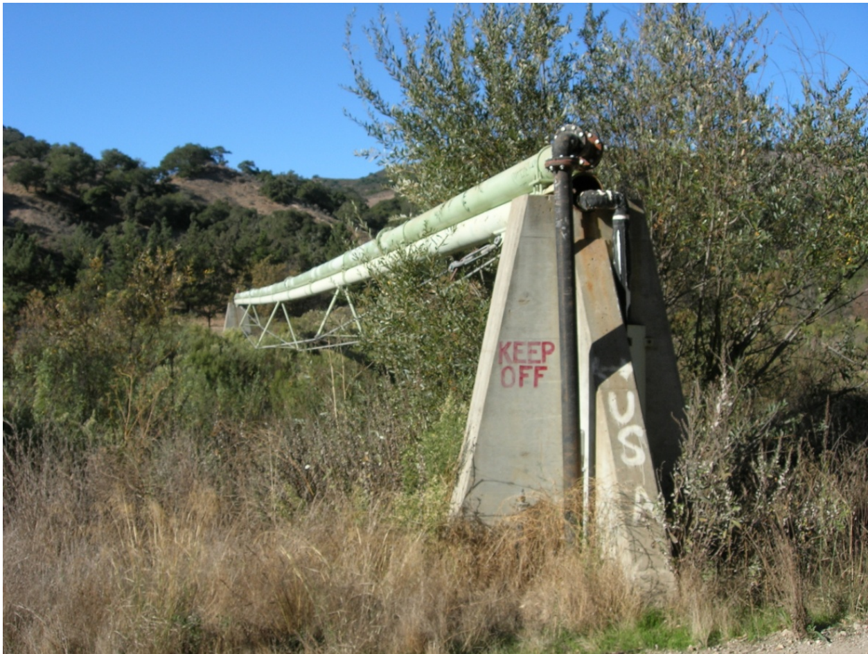
Figure 11: Sewer Force Main Over Wittenberg Creek Arm of Lopez Lake
