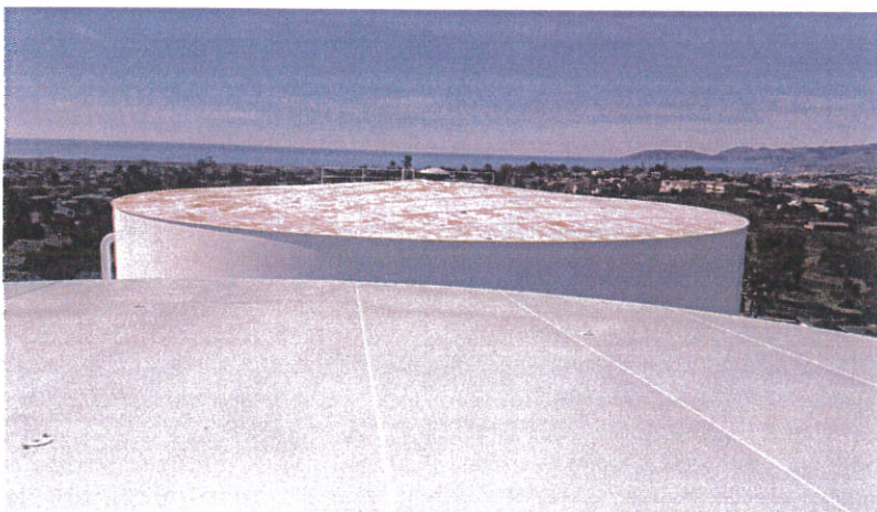
Photo 1: Corrosion on roof of Reservoir 3 (perspective of Reservoir 2)
