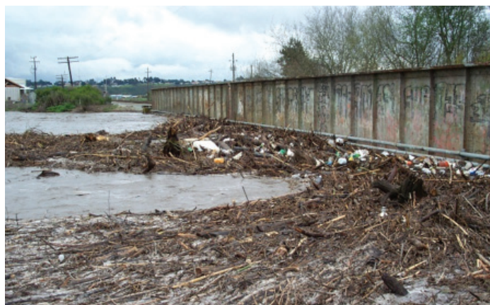
High flows and debris in Arroyo Grande Creek at the railroad bridge (1999 flood event).
