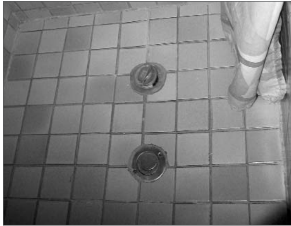
Water inside, reused outside: Dual drains installed in a second-story shower allow water to be diverted to the garden.
