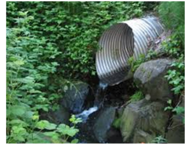
Point Source Discharge Pipeline
