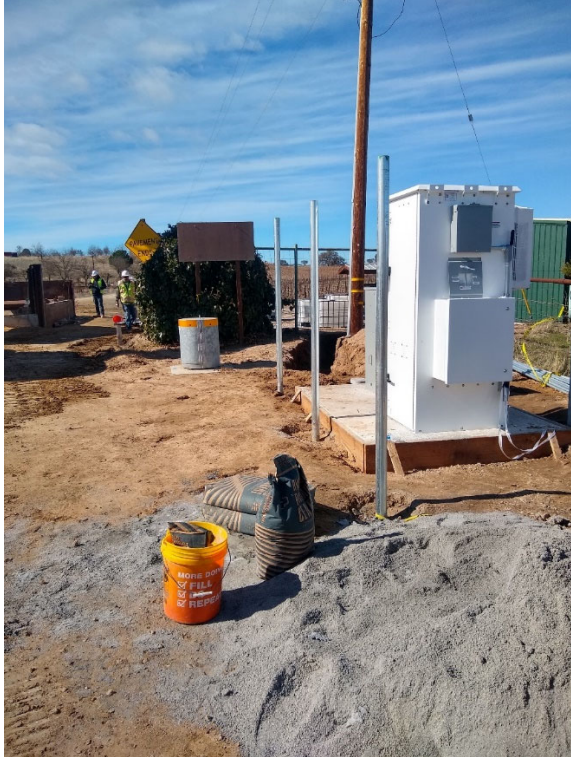
Concrete Pad and Cabinet at Wellsona:
