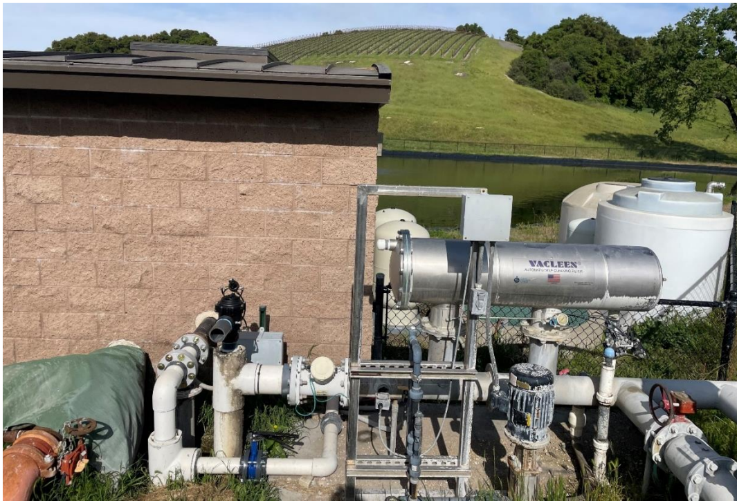
Photo 2. Pump house, booster pump, and filter system.
