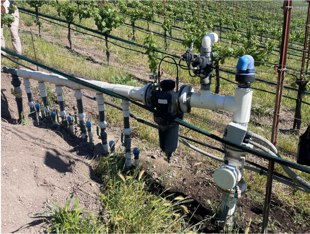
Photo 3. Flow meter at block.
