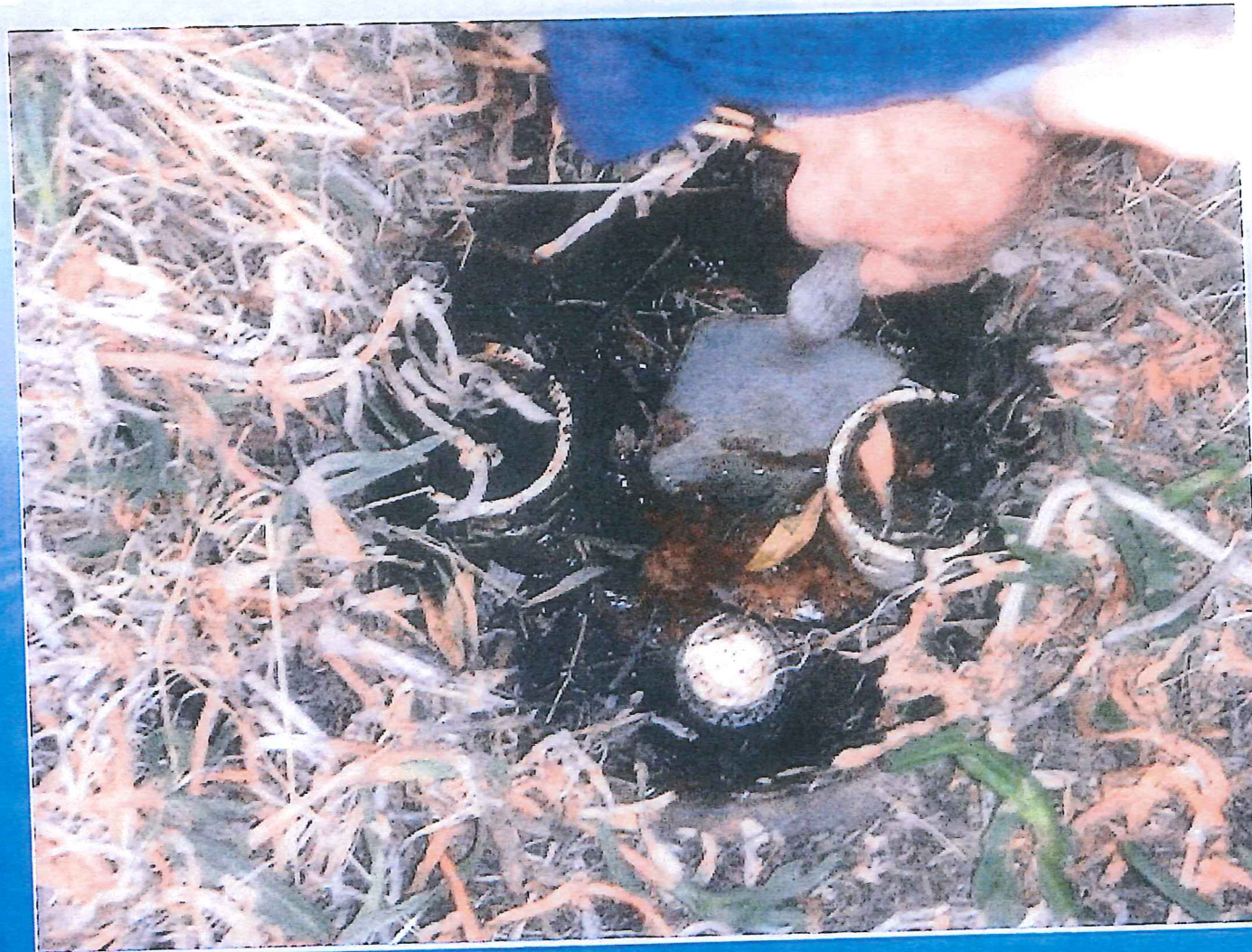
Well in Great Disrepair. Note High Level of Contamination.
