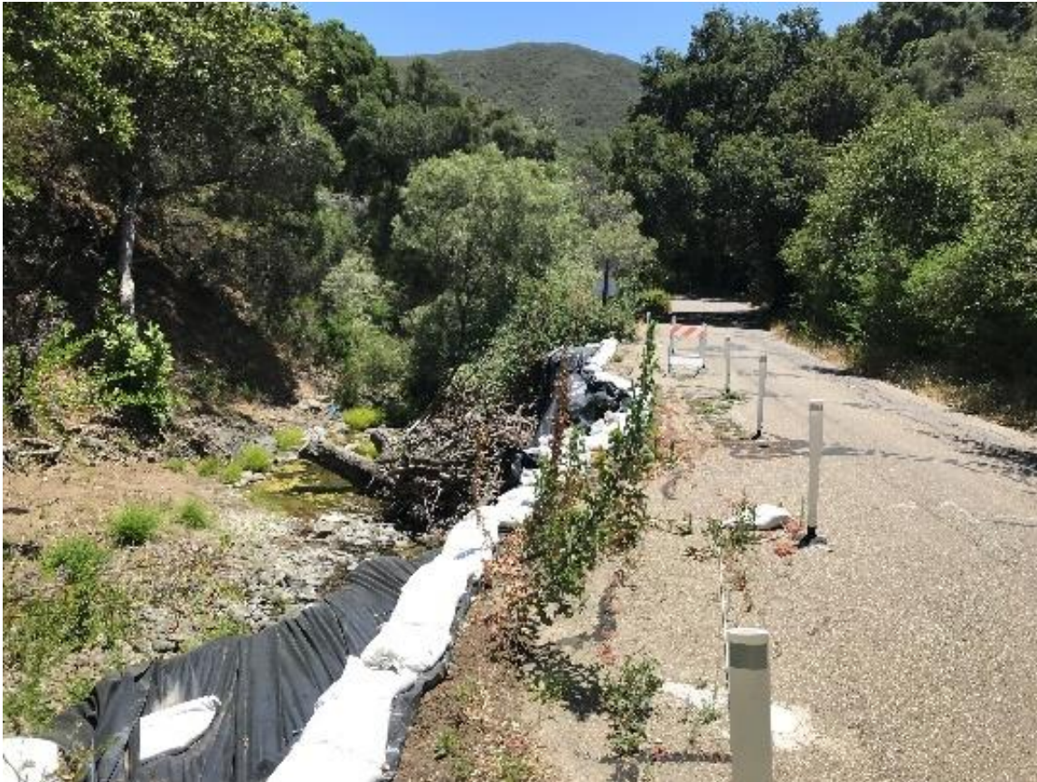
(b) View looking south along project site on Prefumo Canyon Road. Existing fallen tree, to remain, in photograph center.
