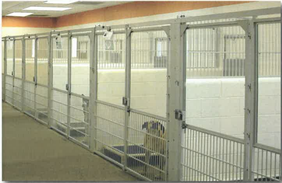
Dog Kennels with upper half in tempered glass allows a clear view of the dogs as the public walks through.
