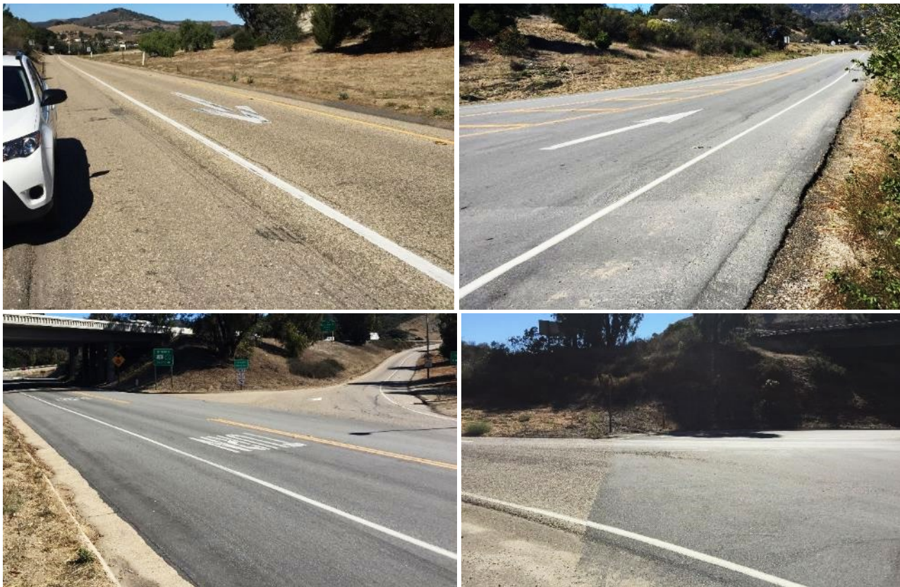
Figure 5: Pavement Conditions: Avila Beach Drive Interchange
