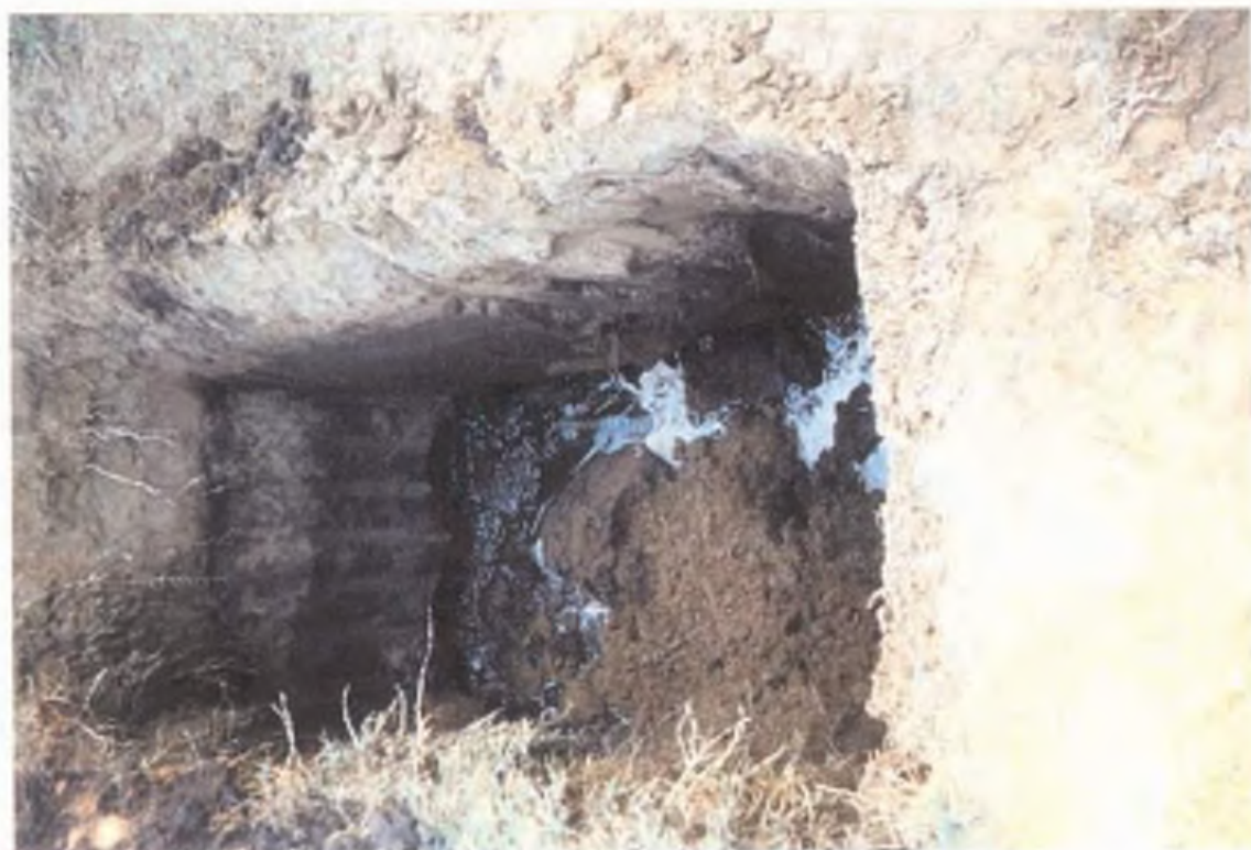
PHOTOS FROM TRENCHING T103-Pismo and 4th Street Los Osos Wastewater Project San Luis Obispo County, California
