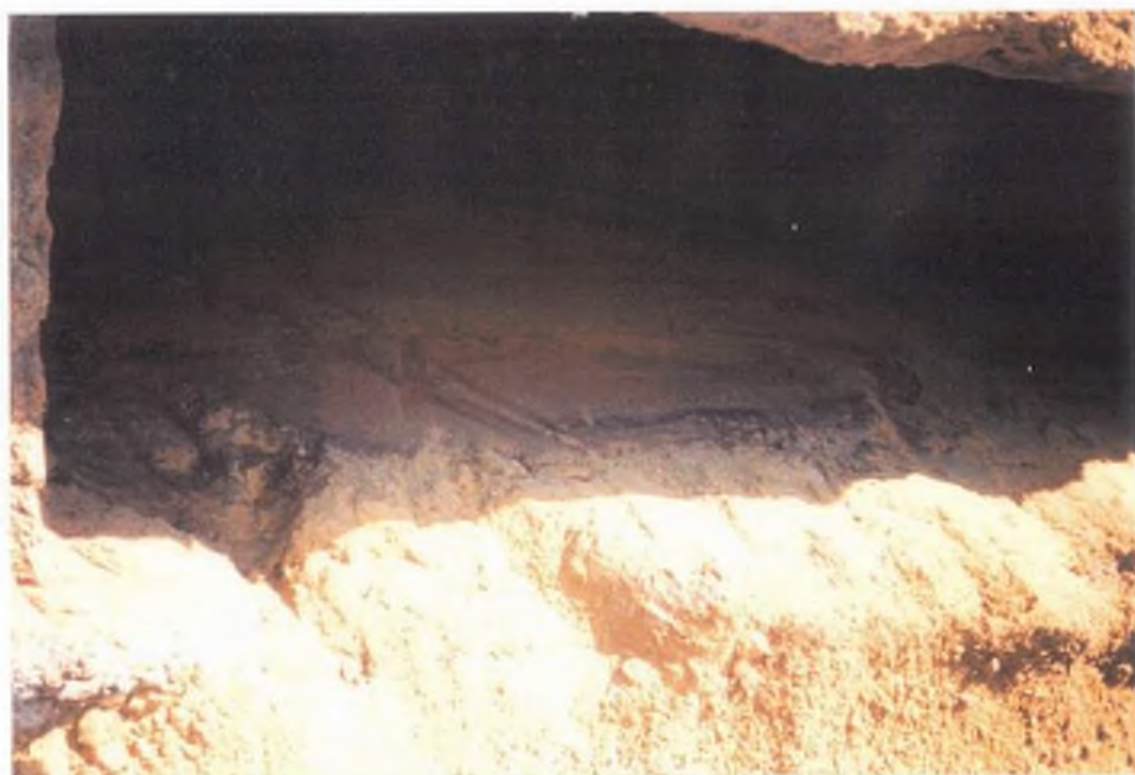
PHOTOS FROM TRENCHING T101-Santa Maria and 10th Street Los Osos Wastewater Project Los Osos, California
