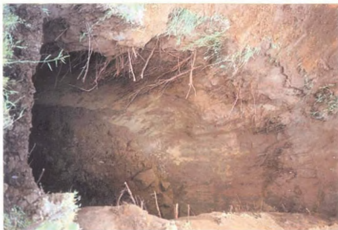
PHOTOS FROM TRENCHING T102-1st Street and Santa Maria Los Osos Wastewater Project San Luis Obispo County, California
