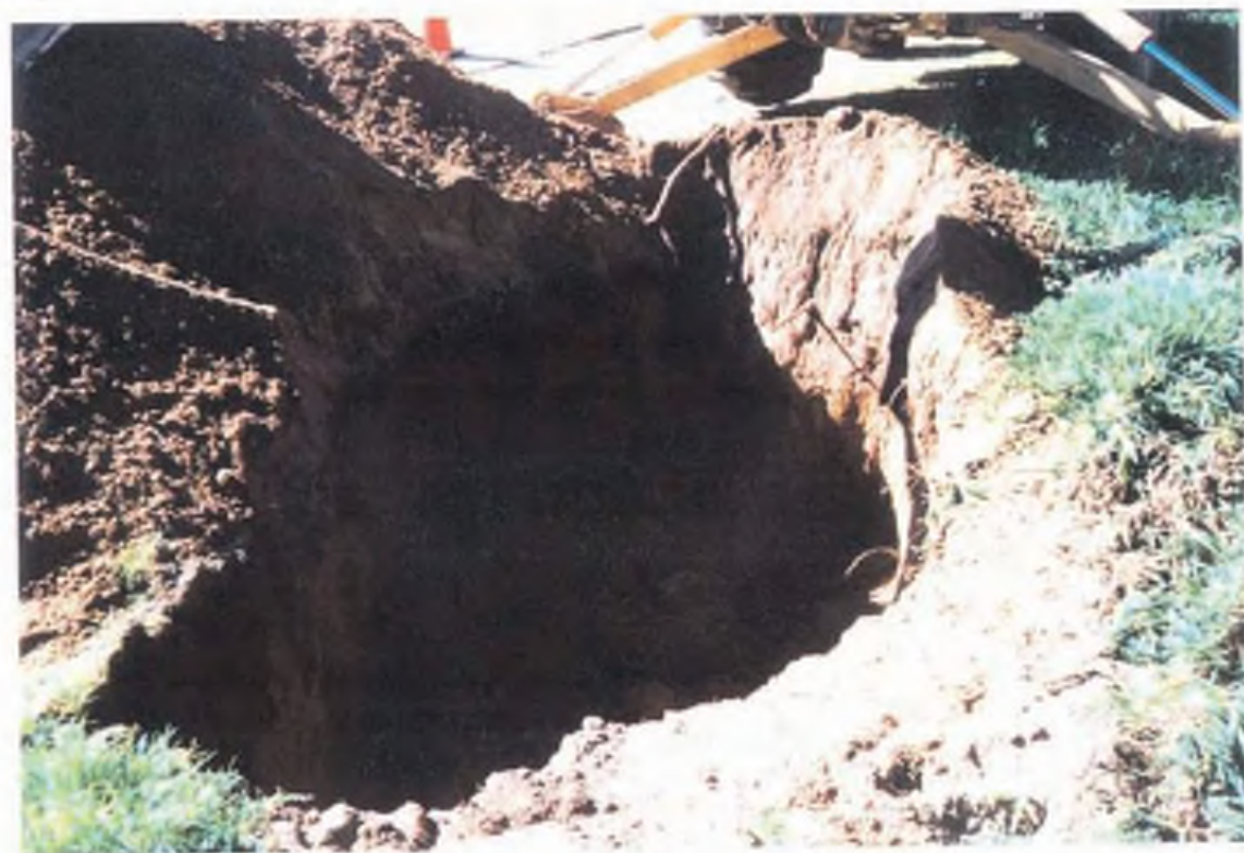
PHOTOS FROM TRENCHING T107-Ramona and 7th Street Los Osos Wastewater Project San Luis Obispo County, California
