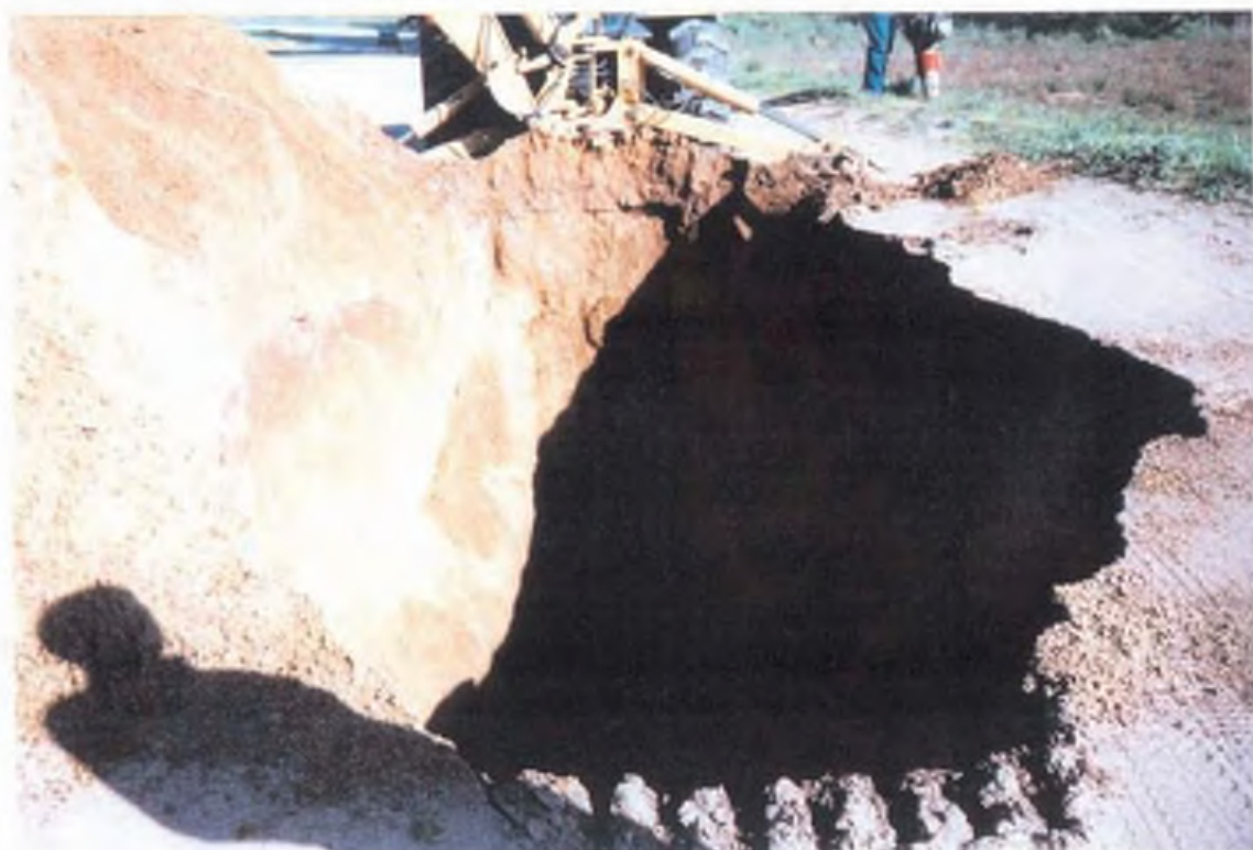
PHOTOS FROM TRENCHING T106-Fairchild and Los Olivos Los Osos Wastewater Project San Luis Obispo County, California
