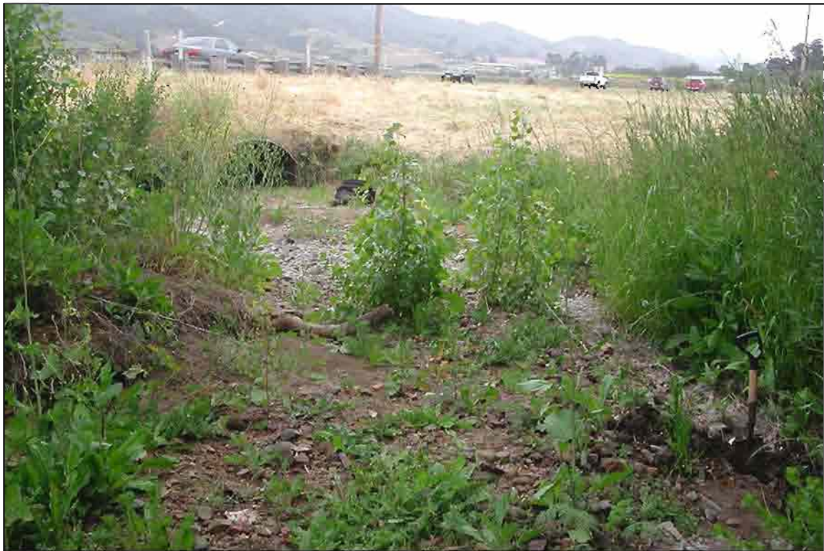
Photograph 20: View of Drainage W-5.a Pit 1, facing southwest toward culvert exiting northern side of Los Osos Valley Road.
