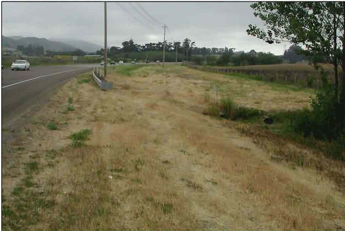
Photograph 17: Drainage W-5.a, from culverts, facing west along north side of Los Osos Valley Road
