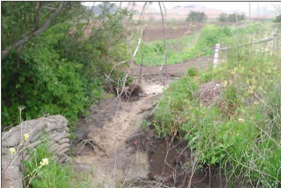
Photograph 16: View of W-5 taken immediately north of Los Osos Valley Road, facing north and downstream.
