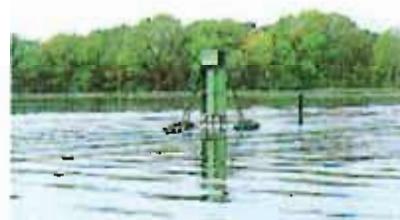
An aerator in the facultative pond
