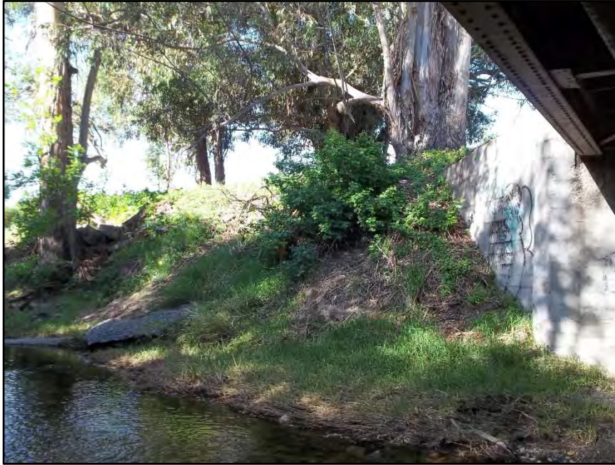
Photo 3. Looking southwest at the existing Bianchi Lane Bridge abutment. This area would be the upstream confluence of San Luis Obispo Creek and the Bianchi Bypass. Creek flows right to left.
