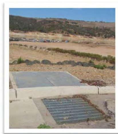
Figure 14: New storm drain with oil separator & rip rap
