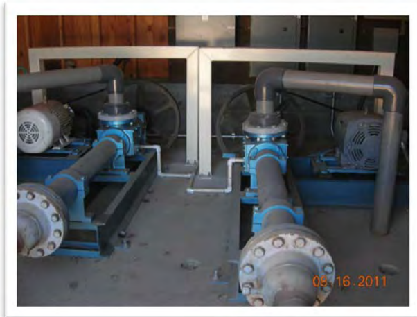
Figure 30: New pump station (Pine Knoll)
