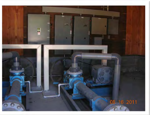
Figure 31: New pump station (Pine Knoll)
