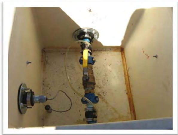
Figure 19: Fuel line sump interior
