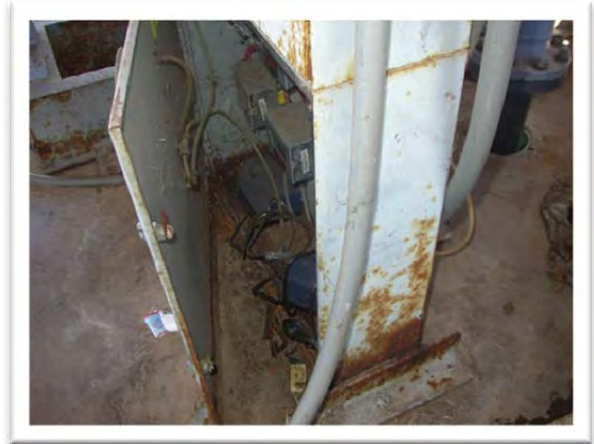
Figure 29: Old pump station (Pine Knoll)
