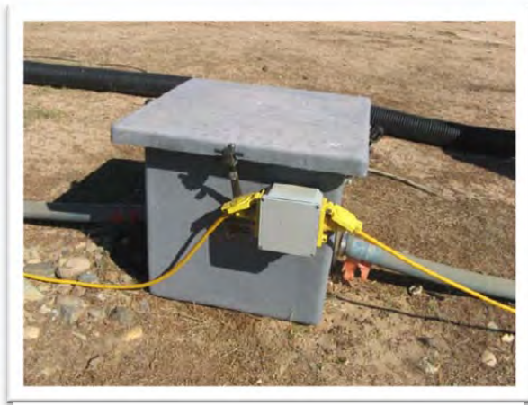
Figure 18: Fuel line sump exterior
