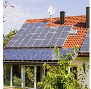
Residential solar panels
