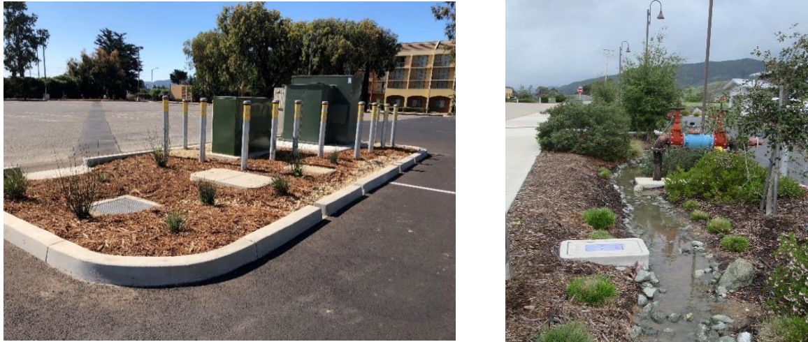
Figure 12: Utility infrastructure in a bioretention feature and obstructing a stormwater swale.
