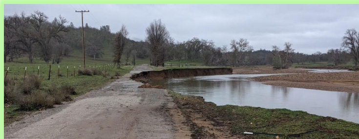
STORM RESPONSE – ROAD WASHOUT, AVENALES RANCH RD, SANTA MARGARITA
