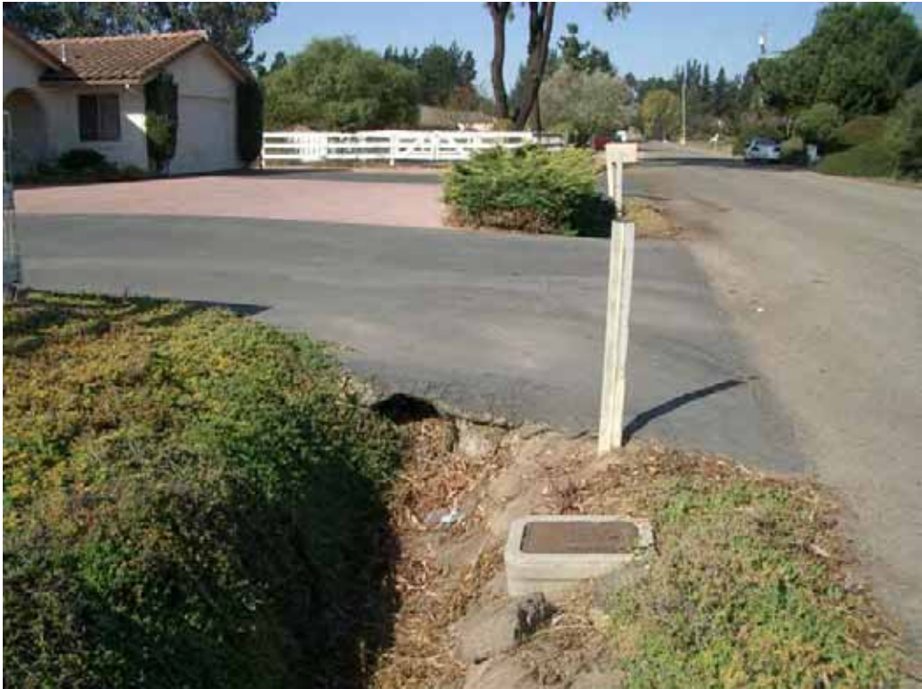
Photograph 3: Culvert on Pablo Lane filled with Sediment. Typical of Culverts in Nipomo.
