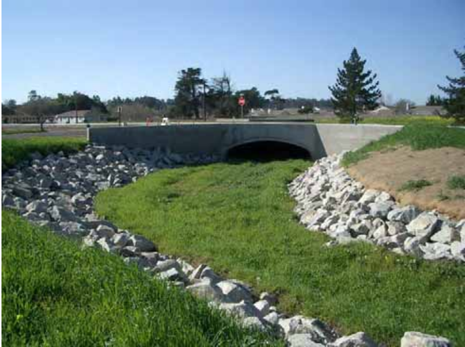
Photograph 15: New arch culvert installed on Haystack Creek at Tefft Street. Installed in 2003.
