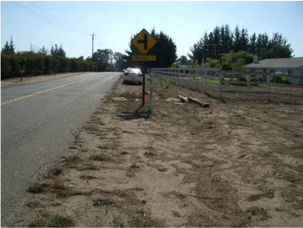
Photograph 4: Division north of Shiffrar. Drop inlet and curb installed on unpaved road shoulder.
