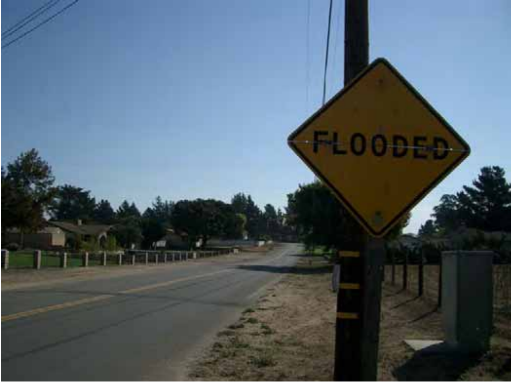
Photograph 1: Location of Flooding on N. Las Flores. Proposed Road Raising Location.
