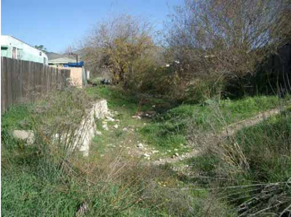
Photograph 13: Overgrown vegetation and channel encroachment on Haystack Creek
