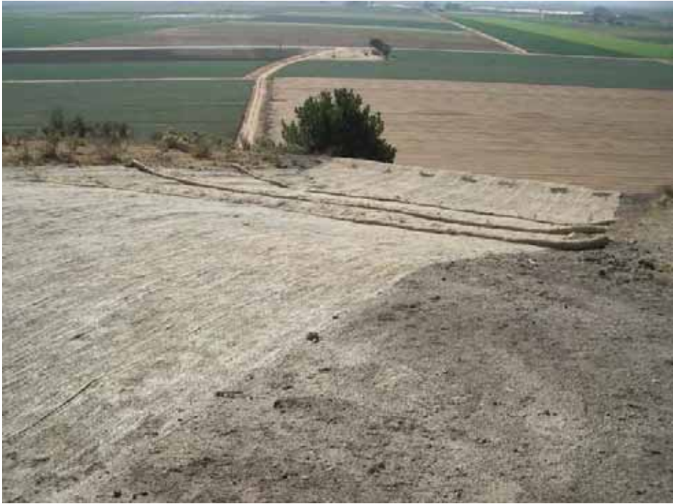
Photograph 6: Erosion Protection of bluff at La Cumbre and Calle Del Sol, completed in fall of 2003
