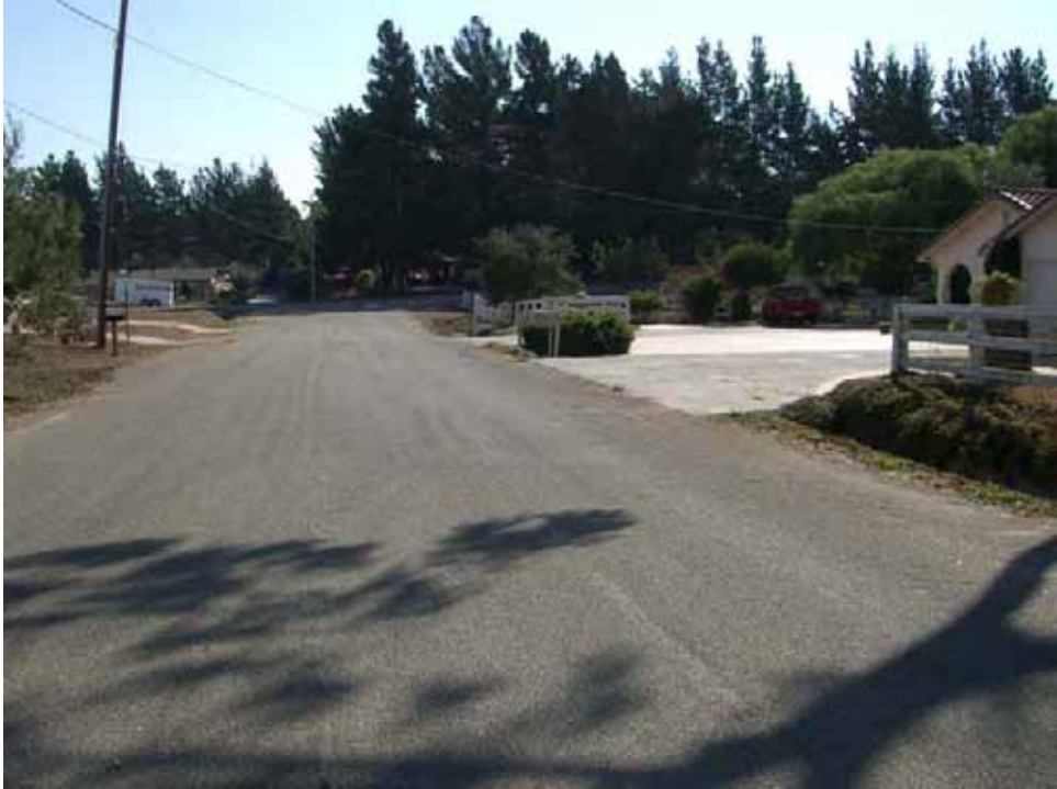
Photograph 2: Location of Flooding on Pablo Lane. Proposed Road Raising Location.
