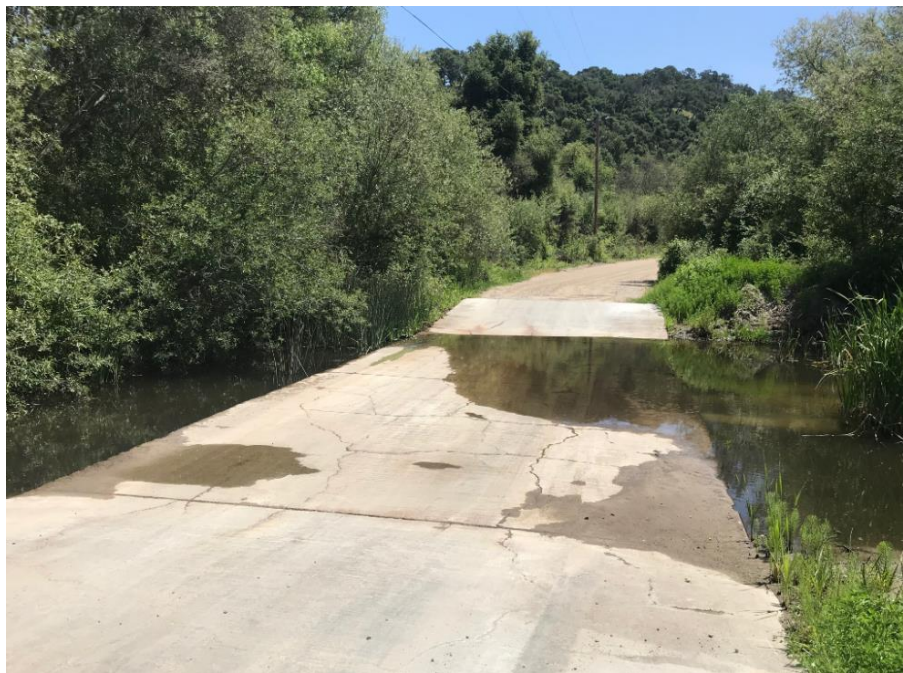
Figure 19: Stagnant water can be seen at a non-flowing Arroyo Grande Creek
