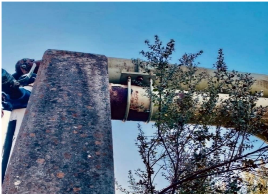
Figure 22: Sewer Force Main Wear or Corrosion
