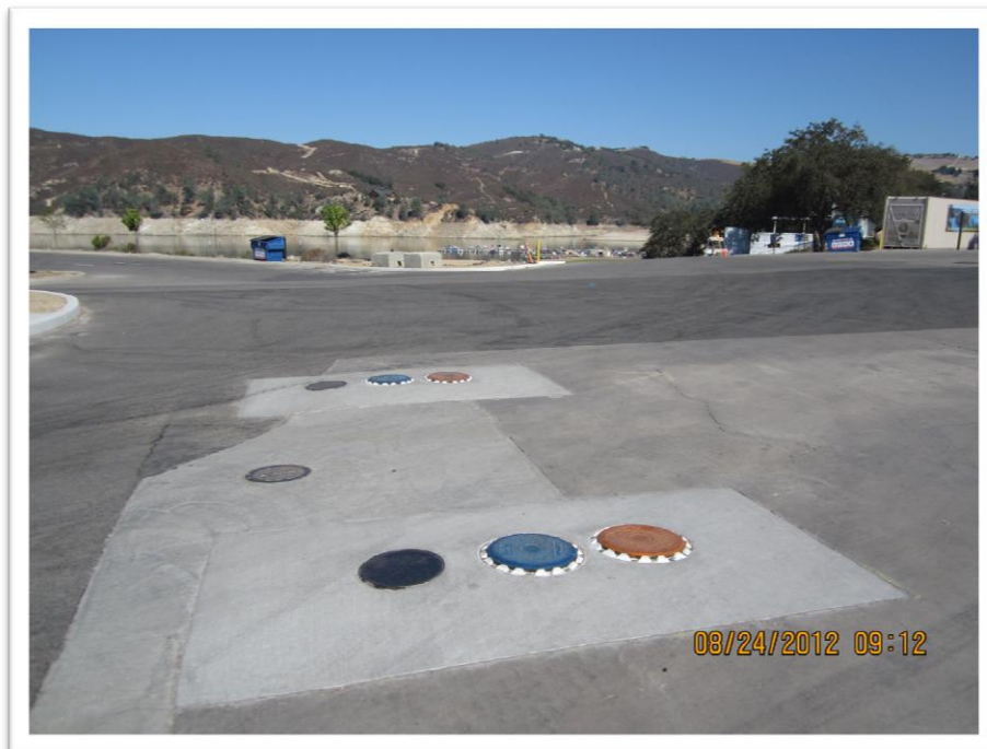
Photo: San Luis Obispo County Public Works Department Figure 77: Underground fuel storage tanks loading ports at Lake Nacimiento Resort
