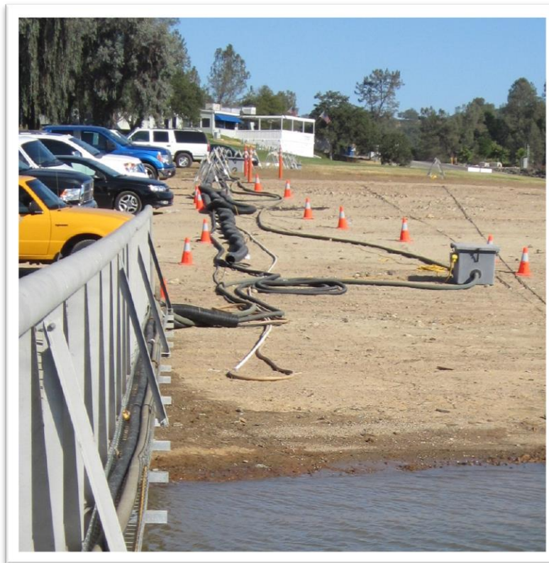
Photo: San Luis Obispo County Public Works Department Figure 79: Lines to run to Lake Nacimiento Resort docks
