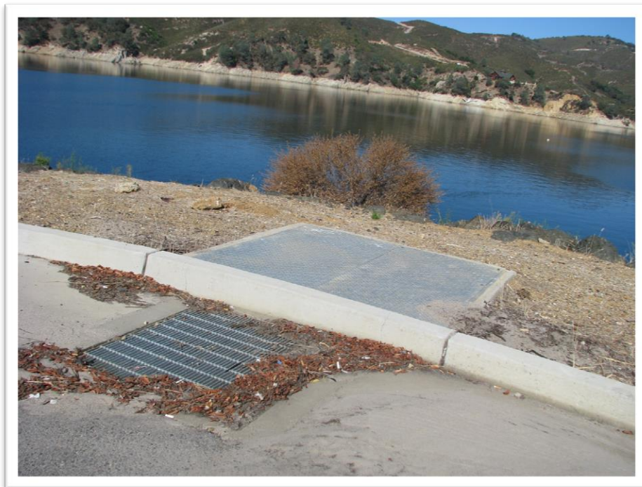
Photo: San Luis Obispo County Public Works Department Figure 56: Storm drain at Lake Nacimiento Resort marina parking lot
