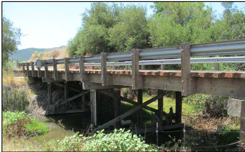
Jespersion Road Bridge over the E. Branch of San Luis Obispo Creek
